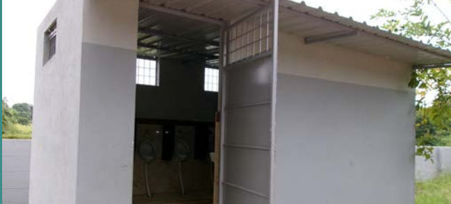
Refurbished Government Higher Primary School (GHPS), Honnenahalli — enhancing hygiene and infrastructure with a new toilet block and a fresh coat of paint.
